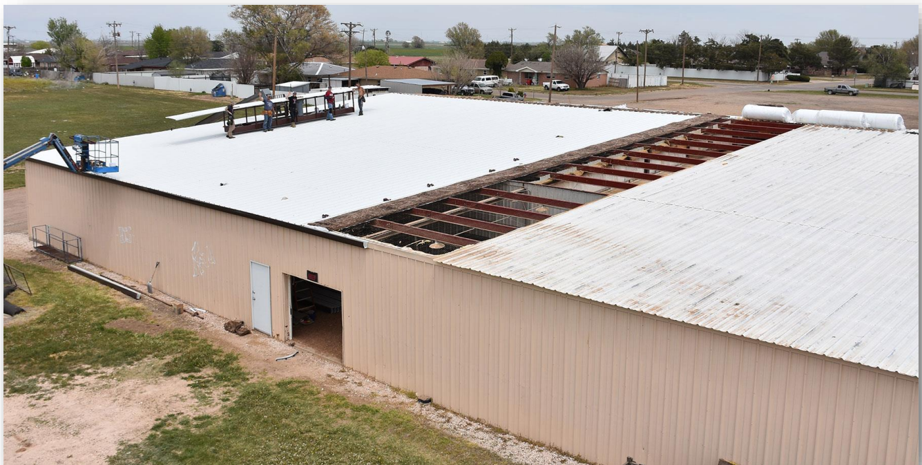
The picture above shows the crew from Hamilton Steel & Concrete working hard on the new roof of the Friona Community Center. You can see the difference between the new and old roof.
