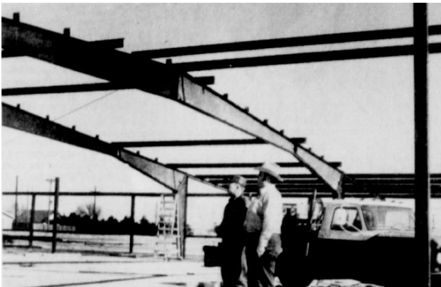
December 9, 1973: Delton Lewellen, left, and Carrol Gatlin watch as the steel and siding begins to go up on Friona's Community Center Center-Showbarn. Photo courtesy of Friona Star
