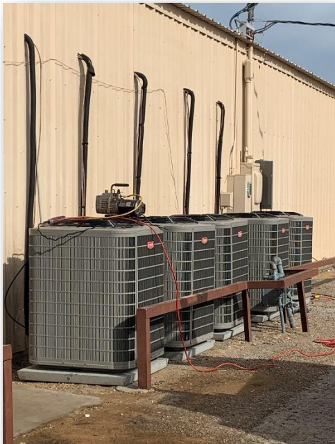
Five air conditioning units were installed to help properly cool the Friona Community Center.
